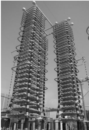
图1 电容器组现场安装图 Fig. 1 Installation diagram of capacitor bank on site
